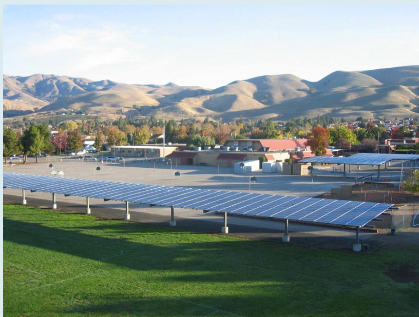
Milpitas Unified School District, PV Installation
