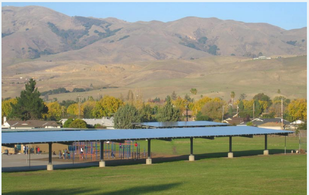
Solar installation at playground area of Robert Randall Elementary School, Milpitas Unified School District
