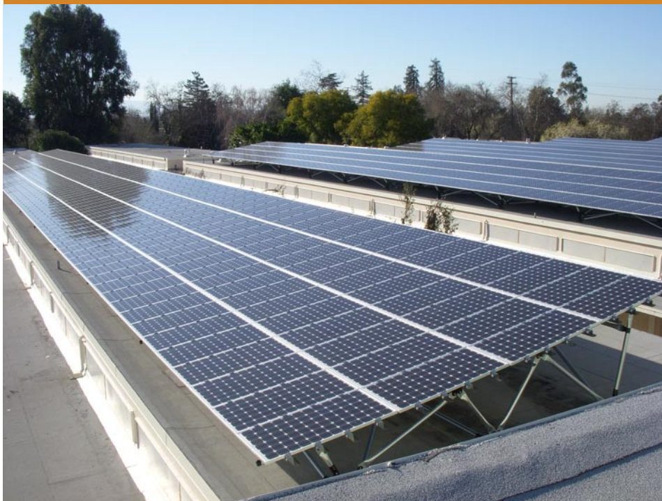
San Jose High School Academy in the San Jose Unified High School District has installed photovoltaic panels on their roof tops.
